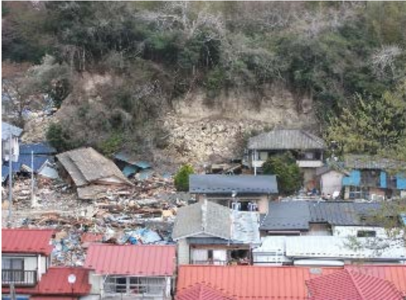
Fig.3 A slope failue in Sabusawa Island (Tsunami from left side also destroyed the houses
